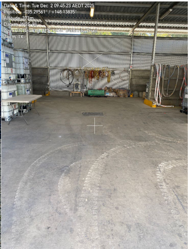
Photo 22 – Dangerous Goods Store. Each segregated area is bunded and has its own containment drain. The drain in the centre has a blind sump, in which any spills can be pumped out.
