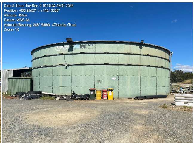
Photo 10 – Part of the WWTP with spill control station.
