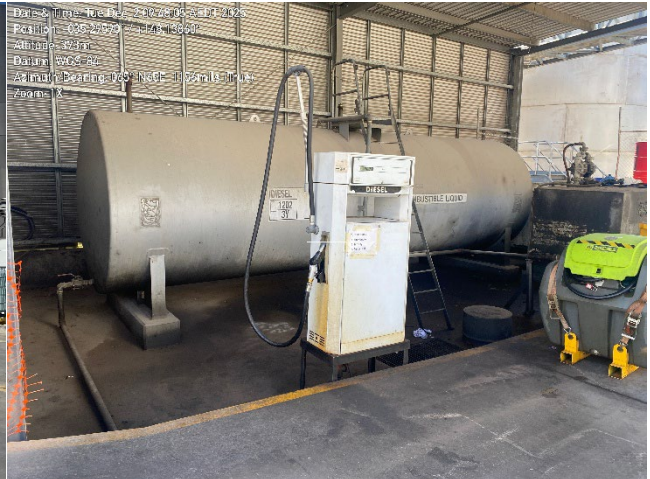
Photo 6 – Bunded diesel storage and bowser.
