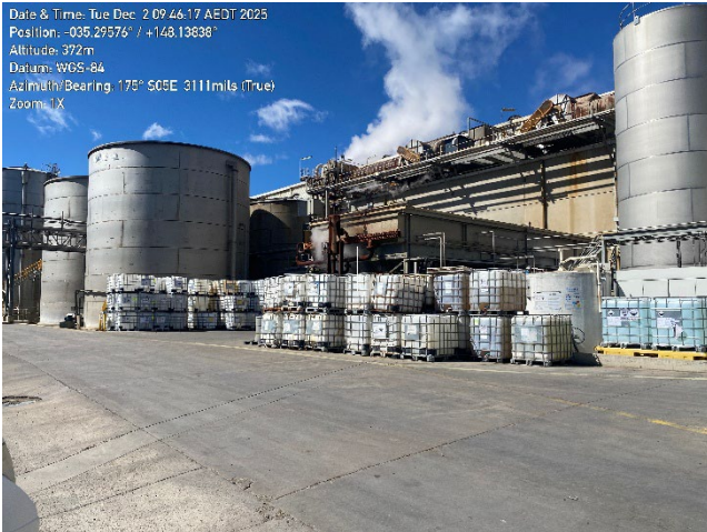
Photo 5 – Bunded chemical storage. Stormwater captured in WWTP.
