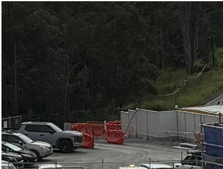
Photo ID: 10 – Further fencing observed at the Site.
